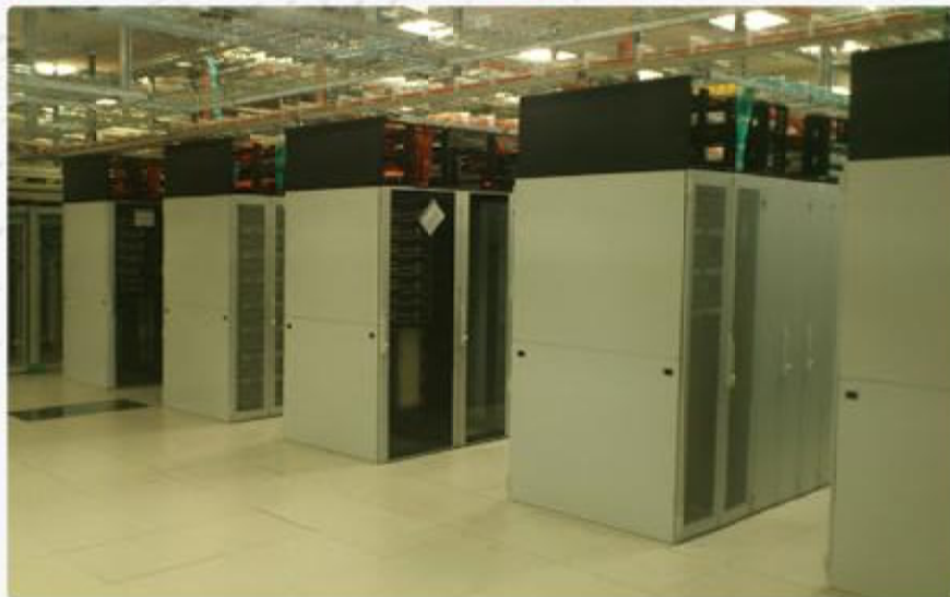
Mellat Bank Main Datacenter 1 MW IT Load
