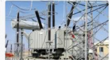
Shoosh 230 kV Substation
