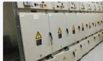
Iran Mall Substation Automation
